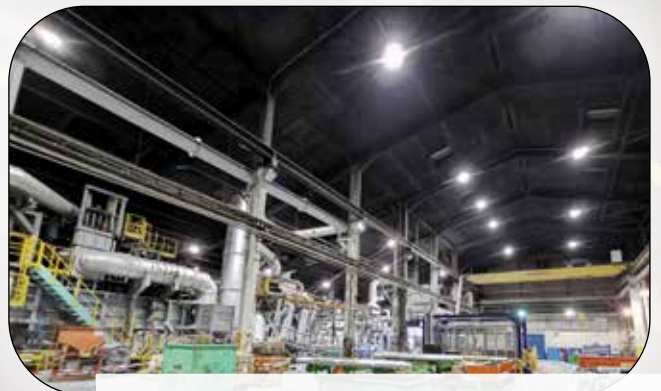
Relighting hall Hydro Aluminium
